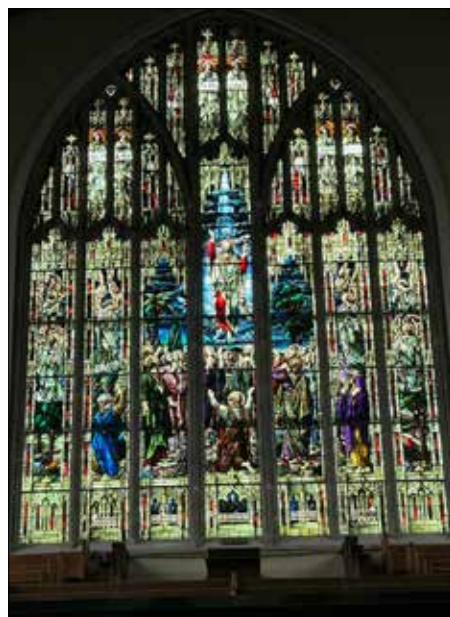
The scaffolding recently came down at Knox Presbyterian Church in Stratford, Ont., as a two-year renovation project to restore the stained-glass windows was completed. For many years, the windows have been dirty and damaged. Despite running into several issues as the work progressed, the beautiful old windows are now available for all to see.
